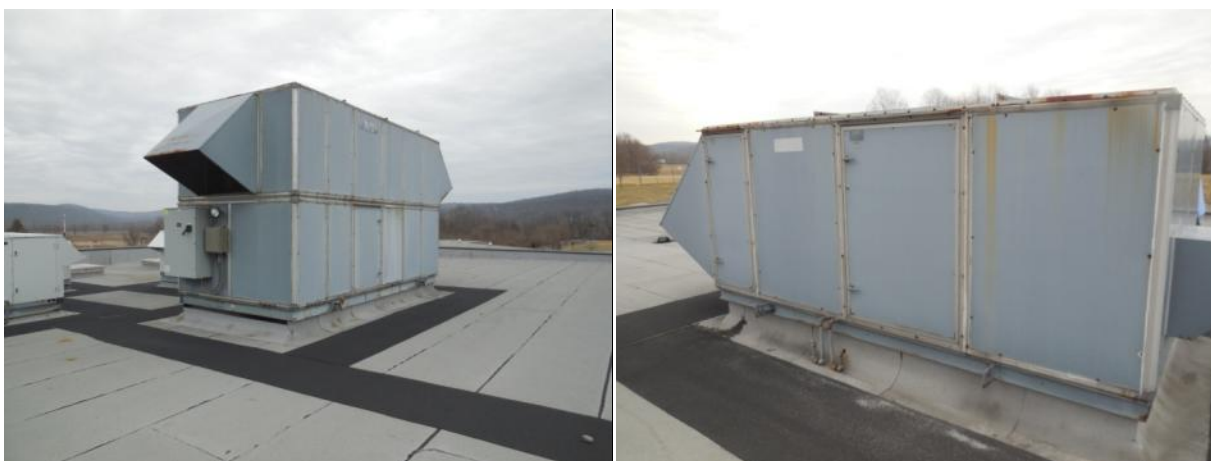
Great Meadows Middle School – Gymnasium and Cafeteria Heat Recovery Units
