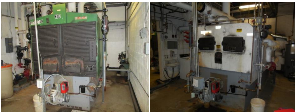
Central E.S. – Weil McLain and HB Smith Steam Boilers
