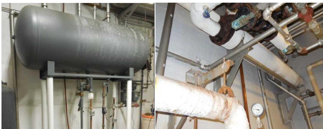
Central E.S. – Condensate Tank and Heat Exchanger
