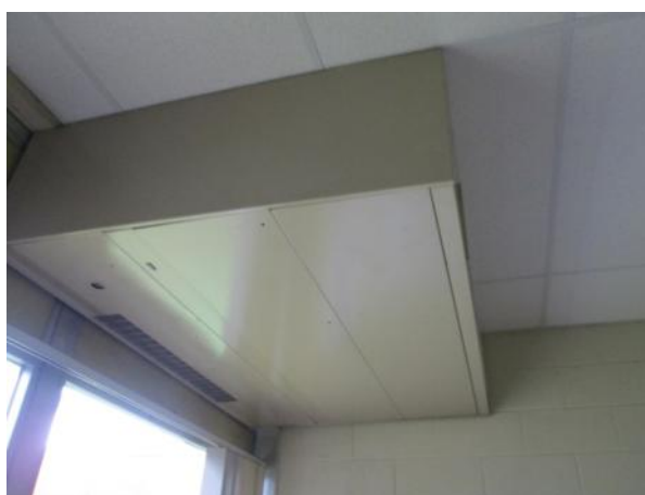
Liberty E.S. – Ceiling Unit Ventilator
