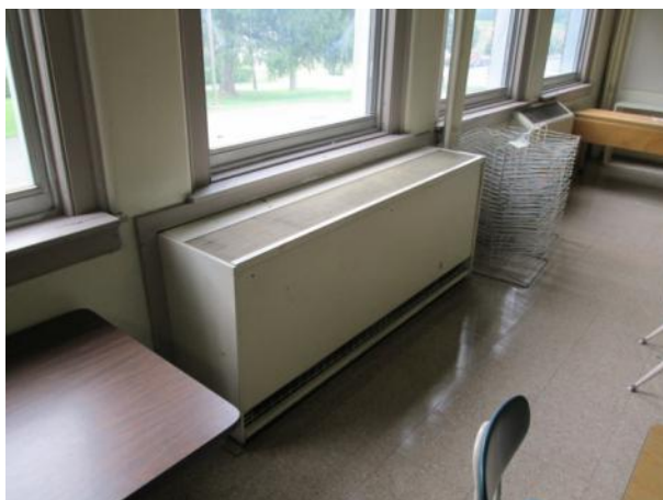
Central E.S. –Unit Ventilator
