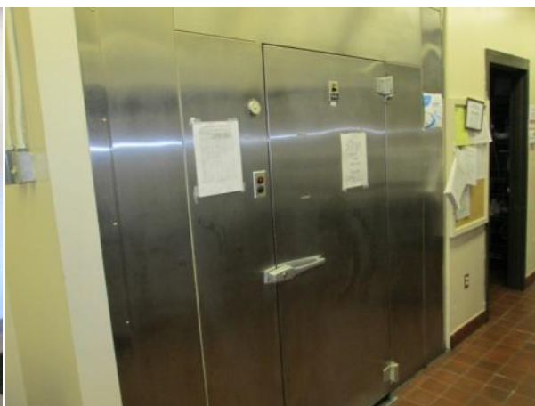
Liberty E.S. – Walk-In Refrigerator and Freezer
